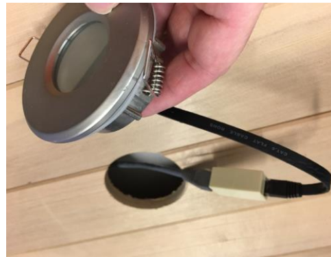
Assembled light fixture plugged in
